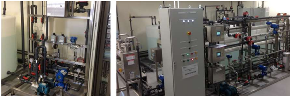
Figure 2.7: Physical process infrastructure and field equipment [180]
